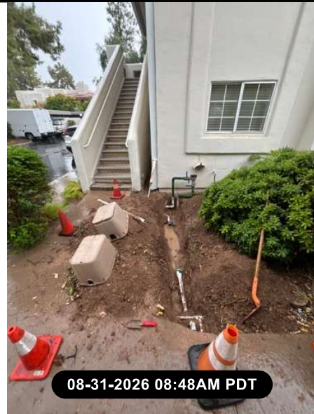
Master Valve and Flow Sensor Install Backflow #1
