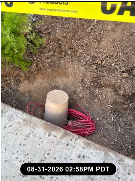
Wire for Master and Flow Sensor Backflow #1
